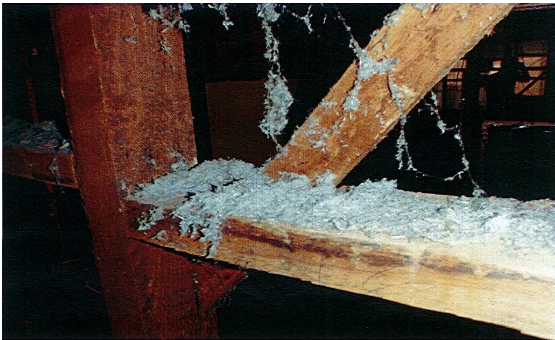
Images of loose-fill asbestos in the living areas of the Downer Home, tendered by Mr Dean Brunton, Hazardous Materials Consultant, Robson Environmental, 17 November 2014.
