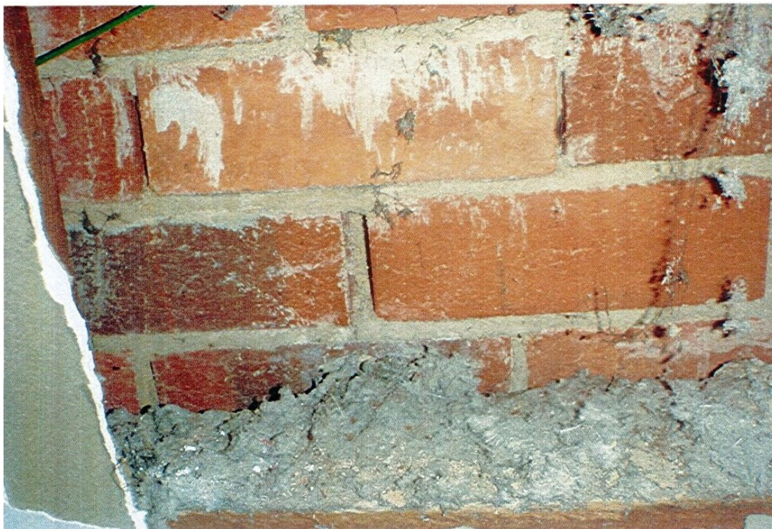
Figure 2 Loose-fill asbestos fibres present on living area bricks in the Downer home
